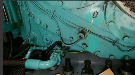
ecoCMS accelerometers retrofitted to GE1.5 MW gearbox
