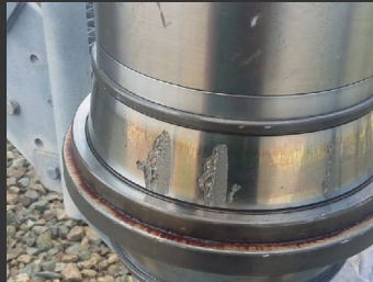
High speed shaft bearing damage detected using ecoCMS
