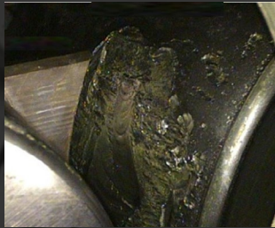
Main bearing macropitting detected using ecoCMS
